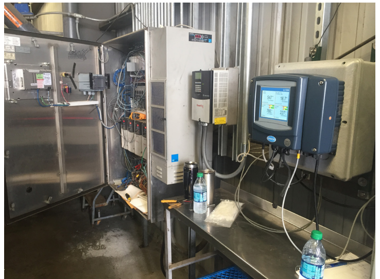
Figure 1: Hach Real-time Control for Sludge Thickening (RTC-ST) installed to help monitor and adjust chemical treatment, pH level and flow in a dairy facility's wastewater treatment plant.
